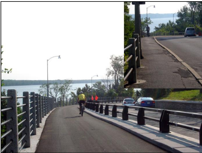
Higher railings along the cliff edge and new guardrail at the roadside grace the beautiful improvements on the Rockcliffe Pathway. Note the increased width compared to the former conditions (inset). Photos: Nancy Biggs/CfSC
